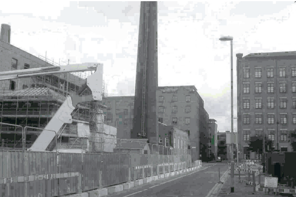
REBUILDING: Investment is turning old industrial centres in Manchester into new luxurious apartments. But but poverty is ever present behind the gloss. Right of page, the 1996 explosion in central Manchester proved a catalyst for change
